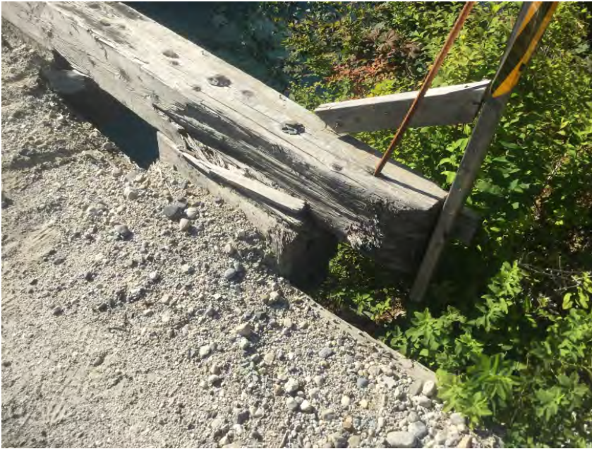
Left Abutment Upstream Corner - Damaged Guardrail & Failed Riser
