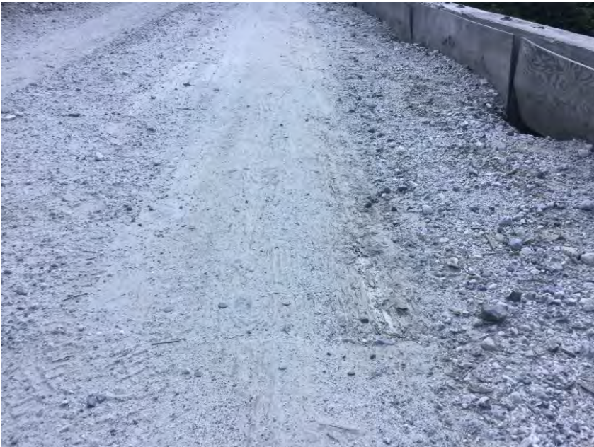
Area of Heavy Wear in Running Planks
