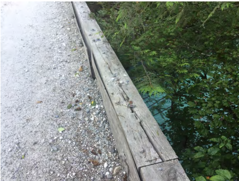
Split Section of Guardrail
